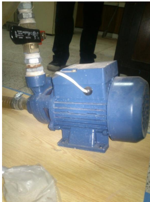
Fig 13 Electric motor to pump the water
