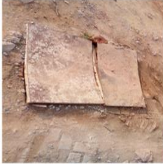
1. Improper Sewage System
