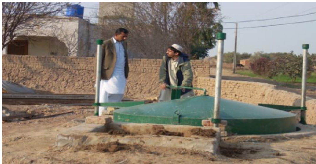
Figure 2: Movable gasholder biogas plant installed by PCRETE
