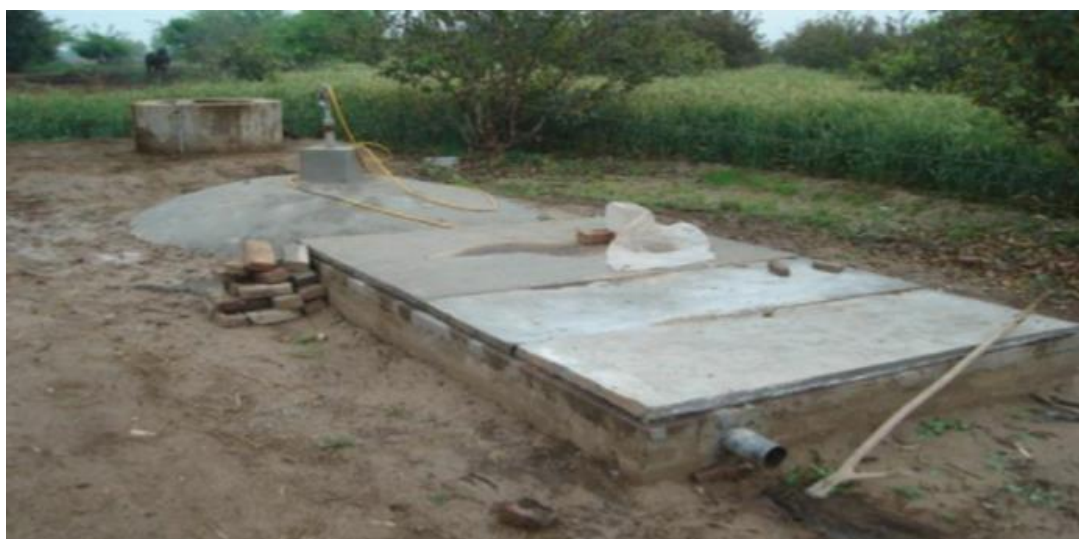
Figure 3: Fixed dome gasholder biogas plant installed by PCRETE
