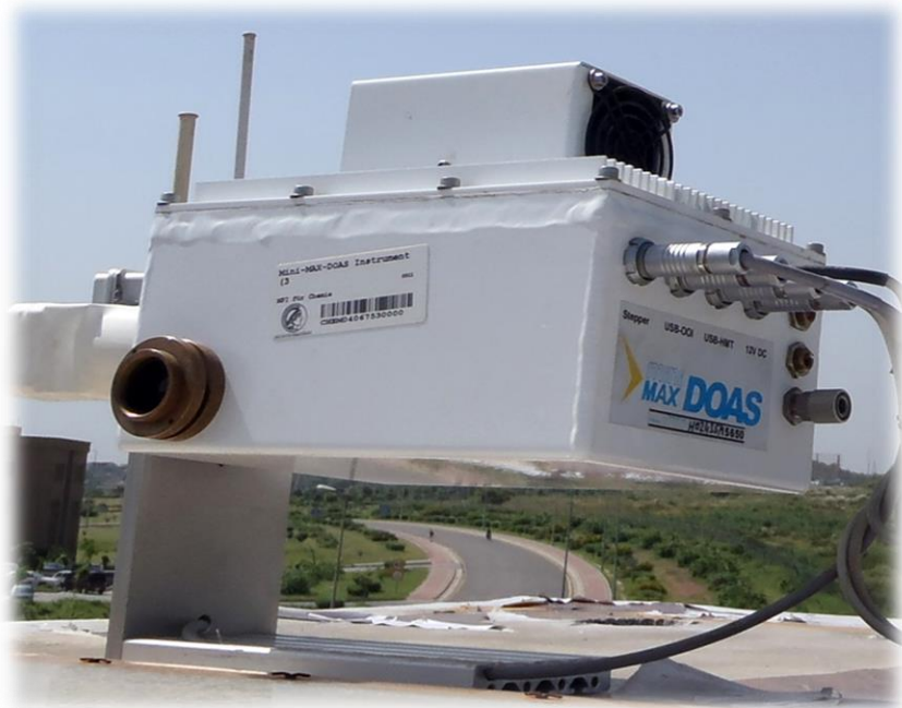
Figure 1.1. MAX-DOAS on rooftop of IESE
