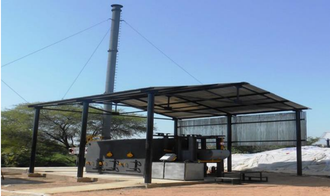
Figure 3.5. Incinerator at site B
