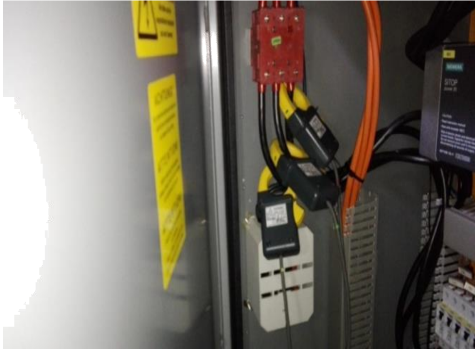
Figure 6 Power Analyzer clamped with main bus of CNC machine
