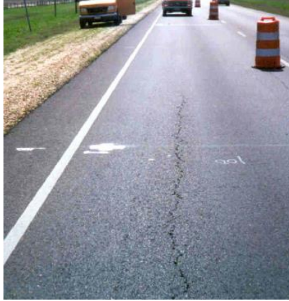
Figure 2. 11 Transverse Cracks in Pavement
