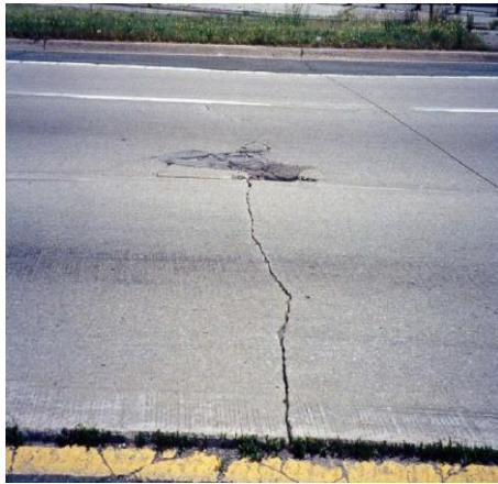
Figure 2. 12 Longitudnal Cracks in Pavement
