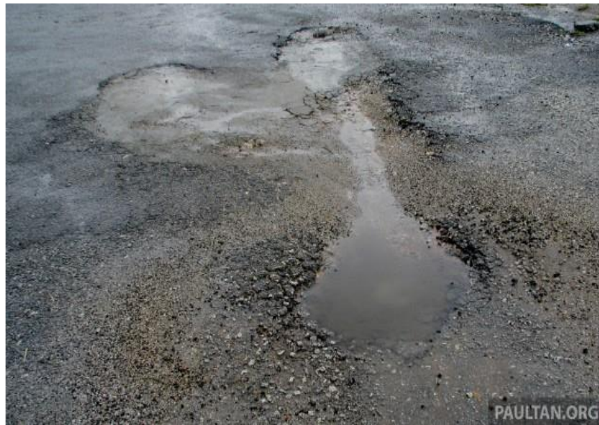
Figure 4: Deteriorated Road Surface
