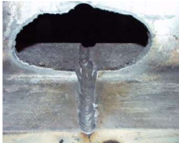
Figure 6: Air arc gouged flange of a beam for Vee and Weld Repair [2]
