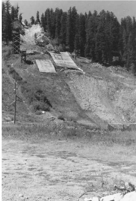
FIGURE 14.14 Howelson Hill sky jump slope failure.
