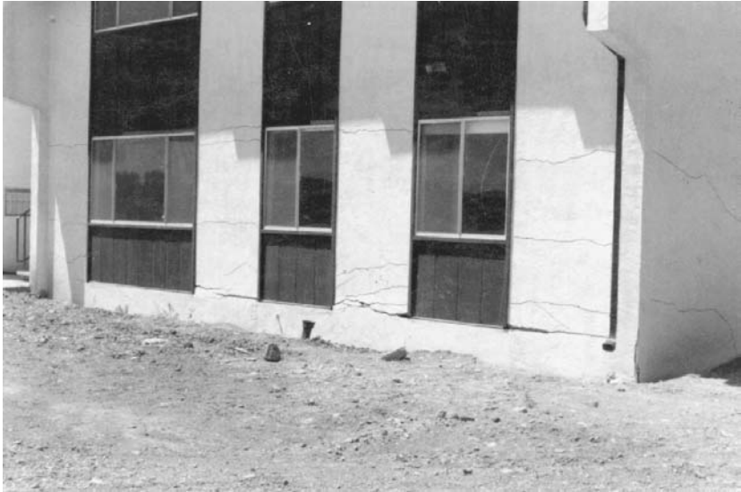
FIGURE 9.2 Typical pattern of cracks due to deep-seated settlement.
