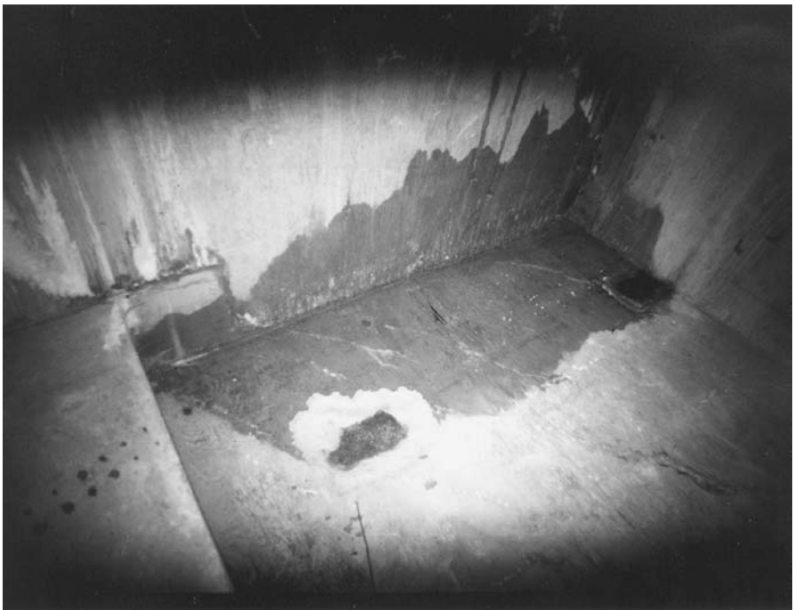
FIGURE 15.1 Water seeped into the lower floor.
