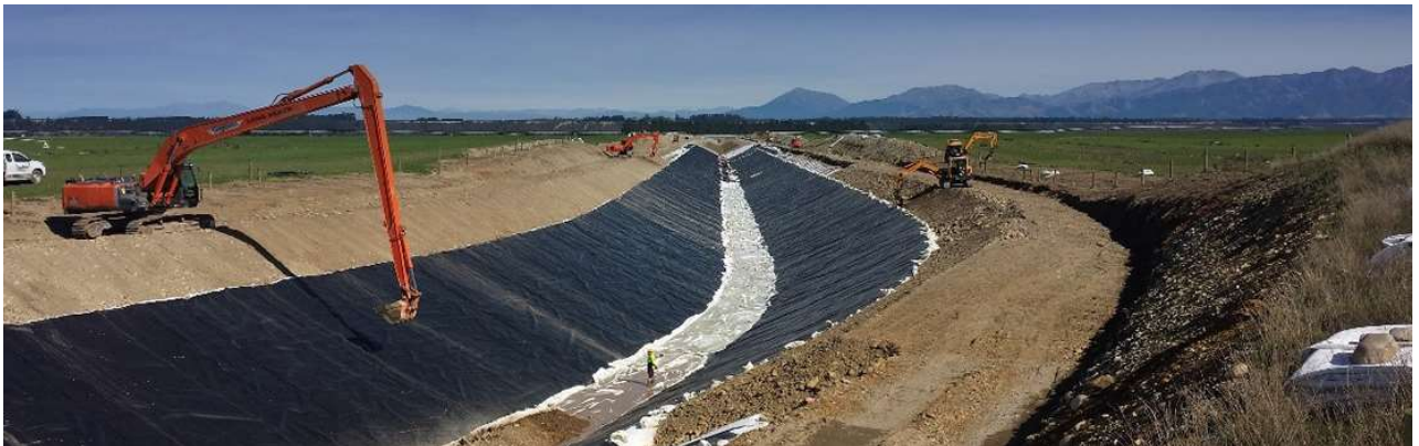
Figure 2.9: Geo-membrane lined canal in New Zealand.
