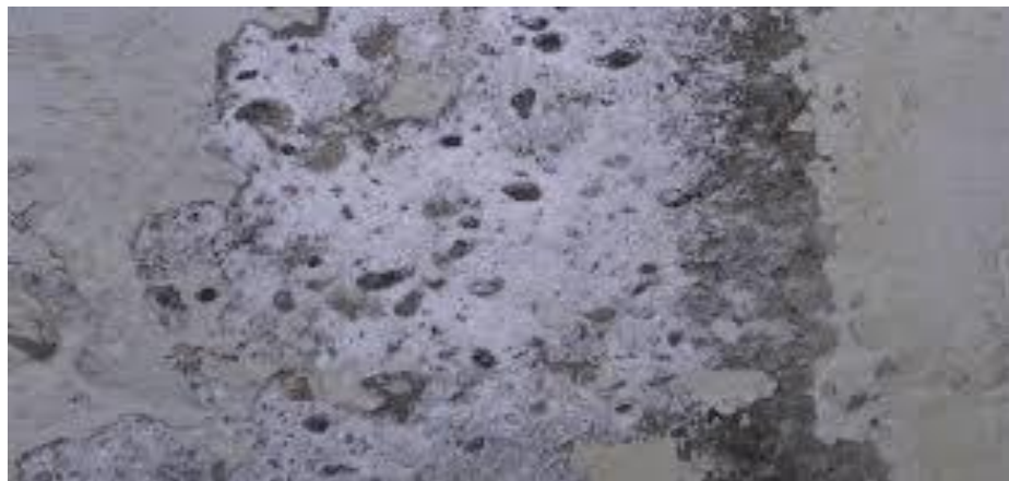
Figure 1: Seepage visible on EOD sidewall
