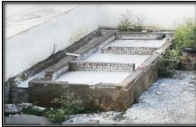
(Figure 8. Sedimentation Tanks)
