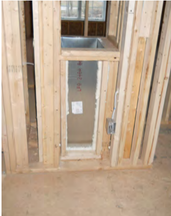
Duct chase between floors.
