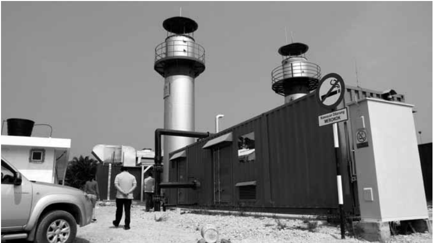
Figure 11.3 The 1 MW Bukit Tagar landfill gas capture plant, Malaysia
