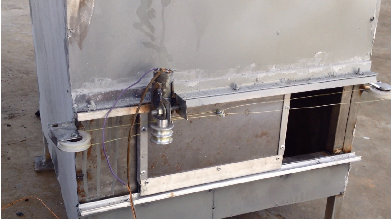
Figure 16 Air Vent Sliding Mechanism
