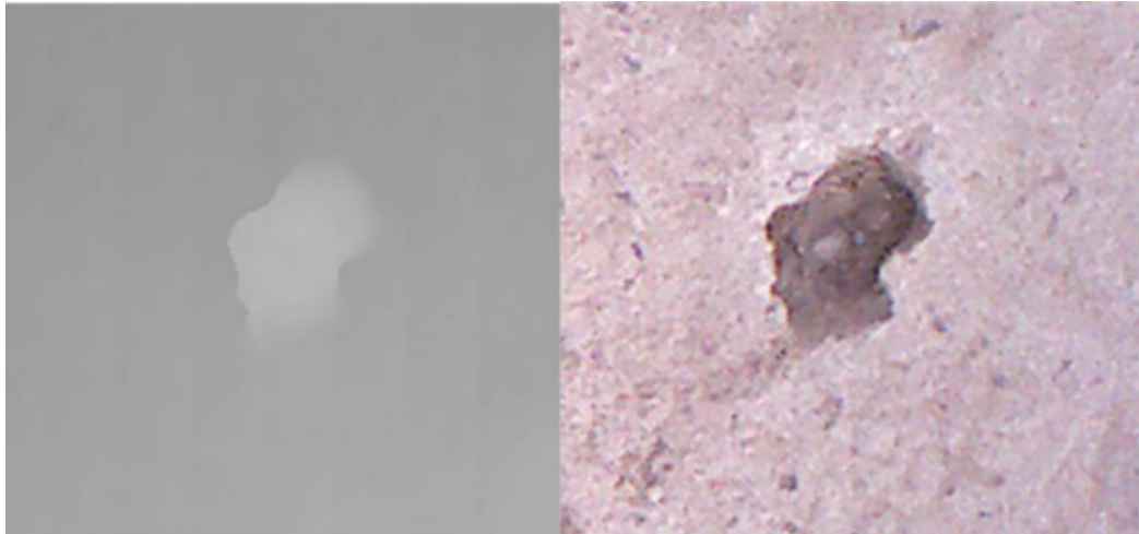
Figure 4.2 : Pothole on the ground for study
