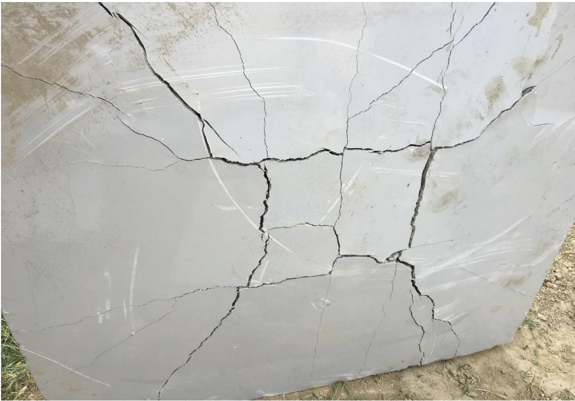
Figure 30: Crack Pattern on Tension Side
