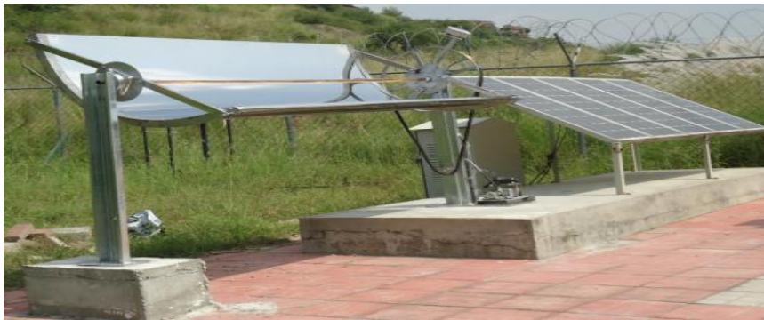
Figure3-2: Parabolic trough installed at NUST Solar Park
