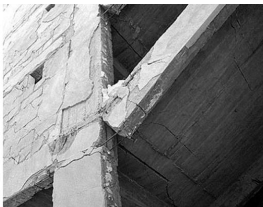
Figure 2.4 A typical failure of Beam-Column joint
