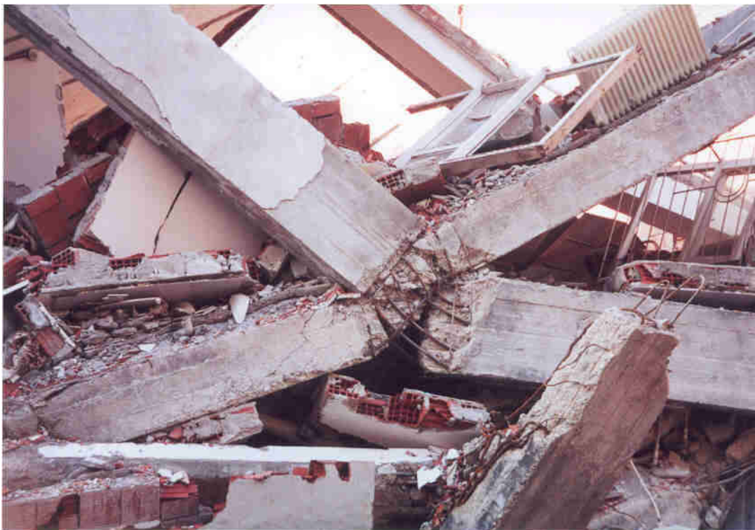
Figure 5: A typical failure of Beam-Column joint
