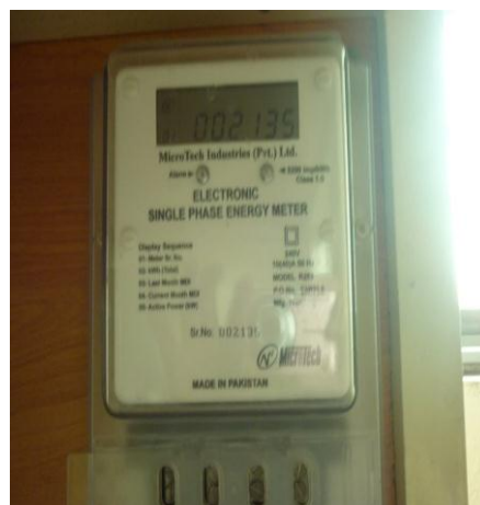
Electricity measuring meter
