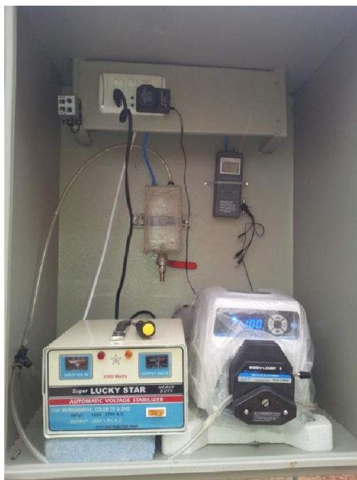
Figure A3: Equipments panel installed on MBST
