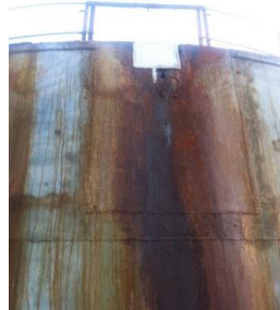
Figure 1: Mild steel tanks corrode in acid storage industries
