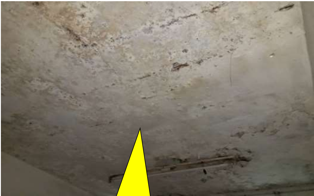
Blistering & Flaking of Paints with Staining
