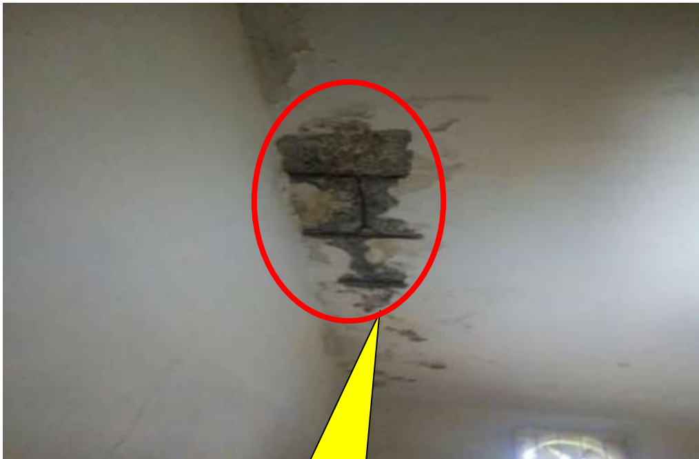
Spalling of Concrete
