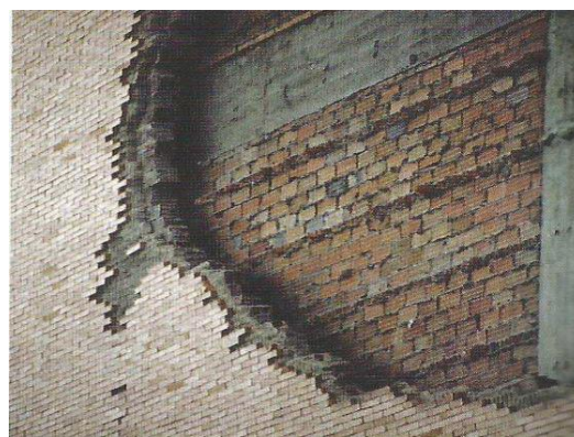
(e) Cladding failure due to moisture/Thermal movement and insufficient ties
