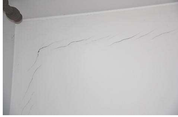
(b) Cracks due to thermal movements
