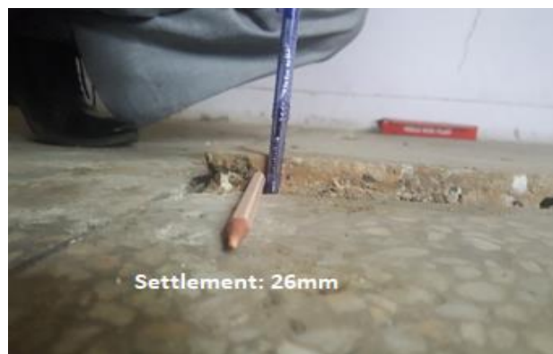
(e) Settlement in floor of Bedroom 2
