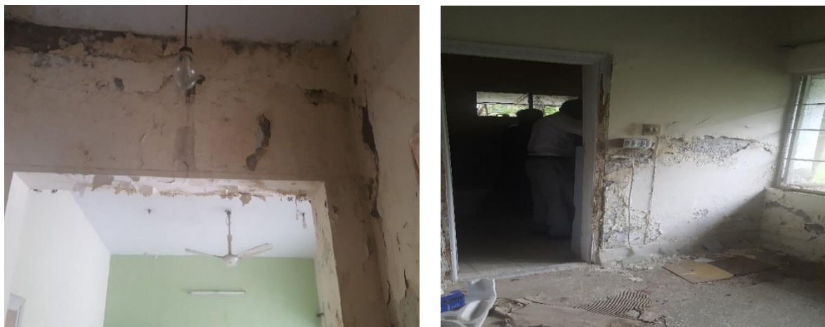
Fig 4.10 Seepage in walls
