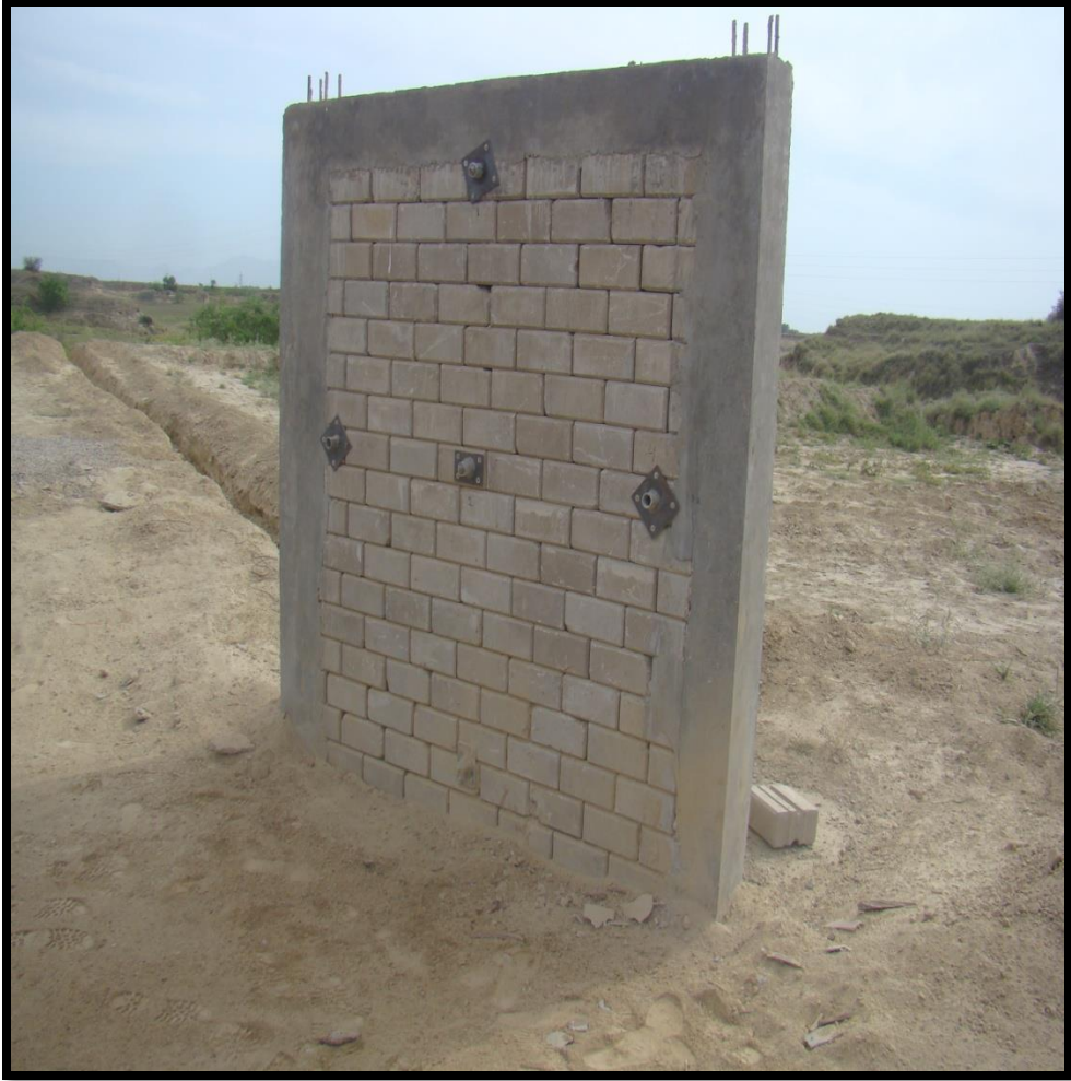
Figure 4. 2 Condition of wall after test # 1
