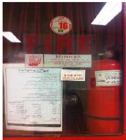
Figure 4.1: Fire extinguisher at hospital A
