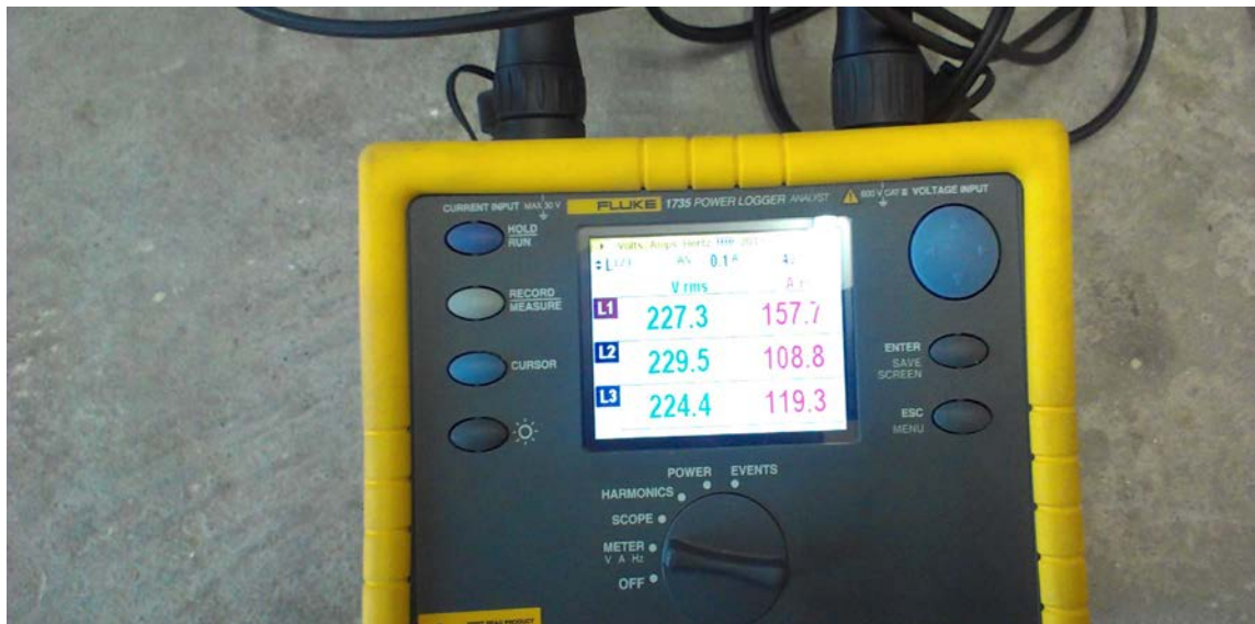
Figure 3-2: Monitoring building load
