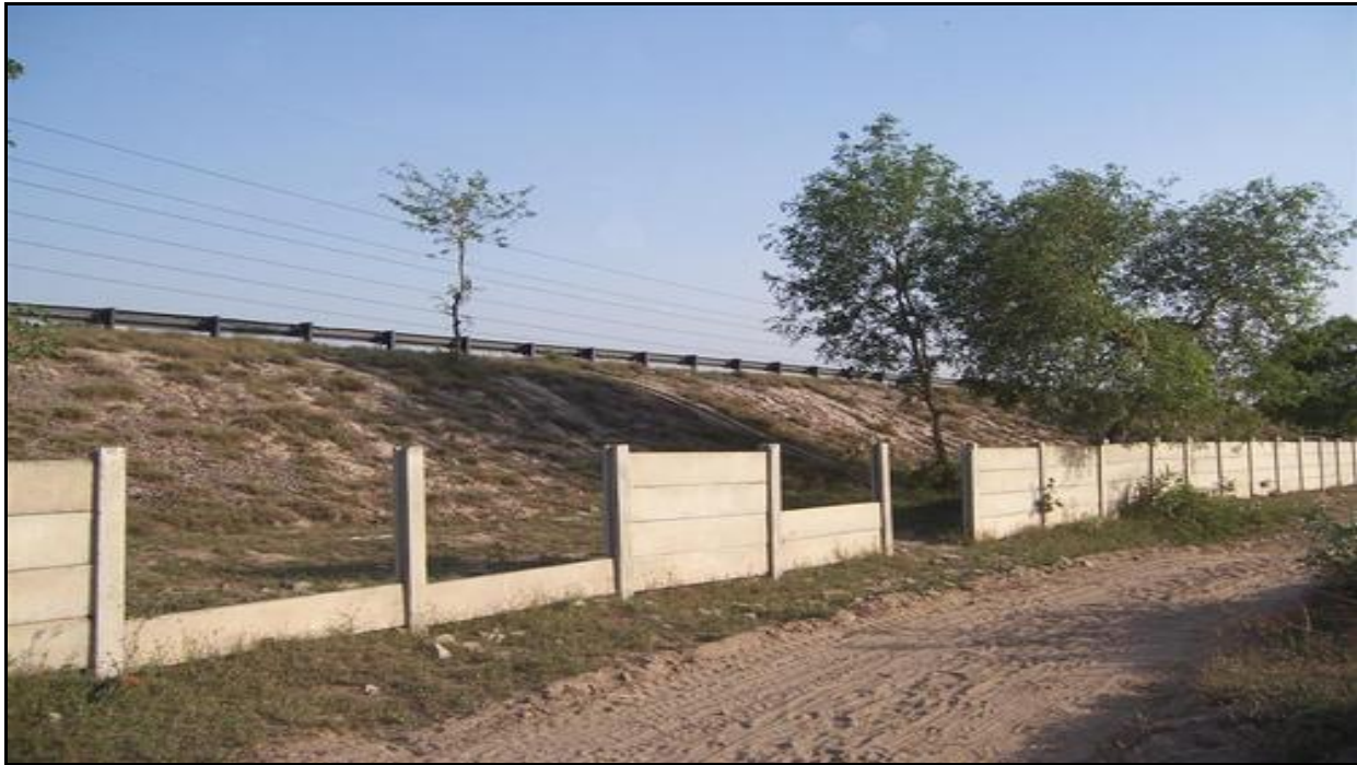
Figure 4.31: Present Condition of Safety Wall Near Lahore (0km-15km)
