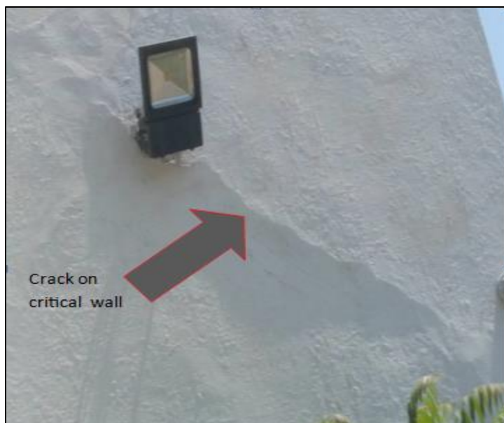
Fig 1.2: Critical wall crack
