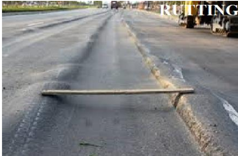
Figure 2.3 Rutting in Flexible Pavements
