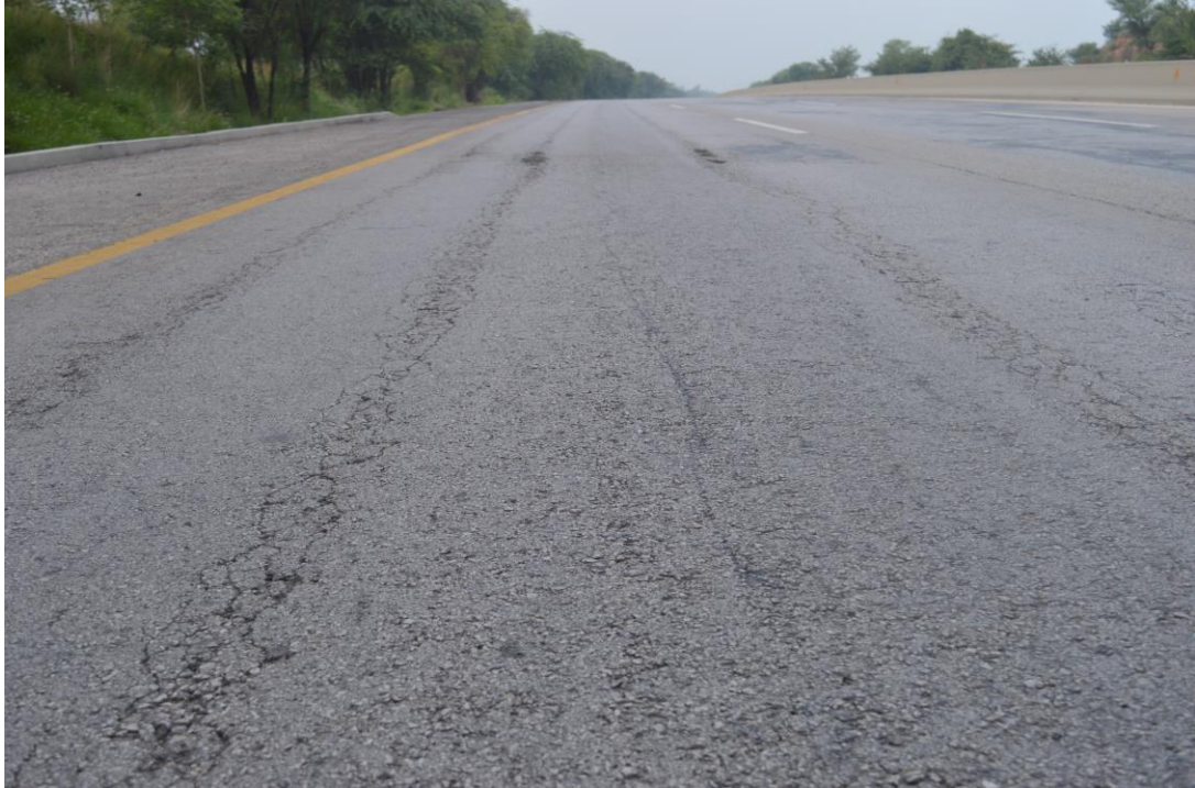
Figure 3.3: Fatigue Cracking on M-2
