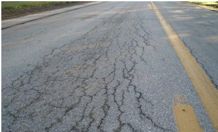
Figure 2.2: Alligator pattern cracking (Miller and Bellinger 2014)
