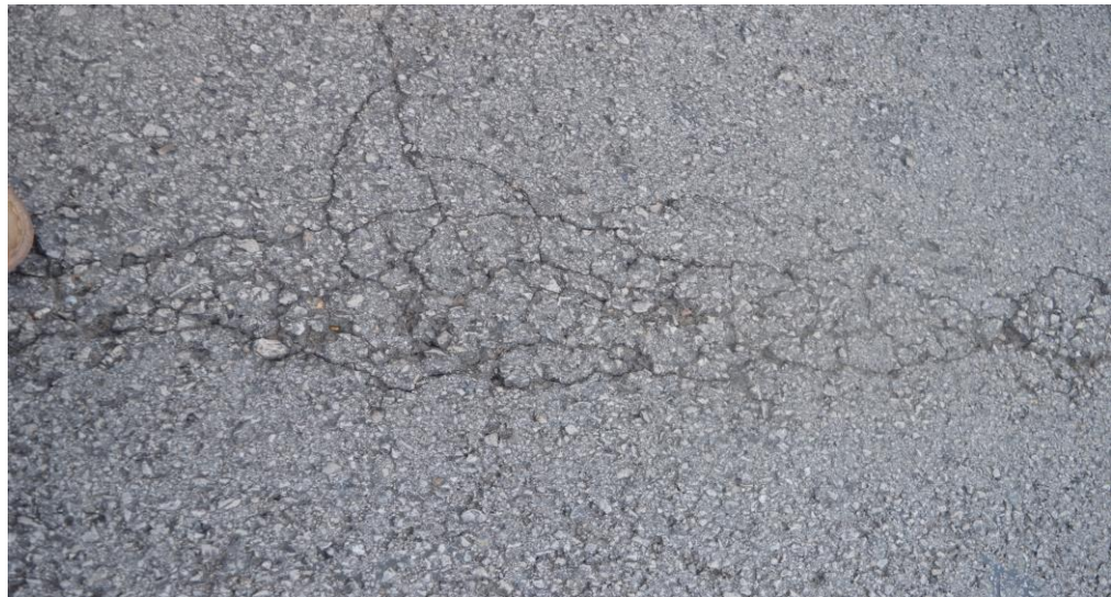
Figure 3.4: Fatigue Cracking (Close View)
