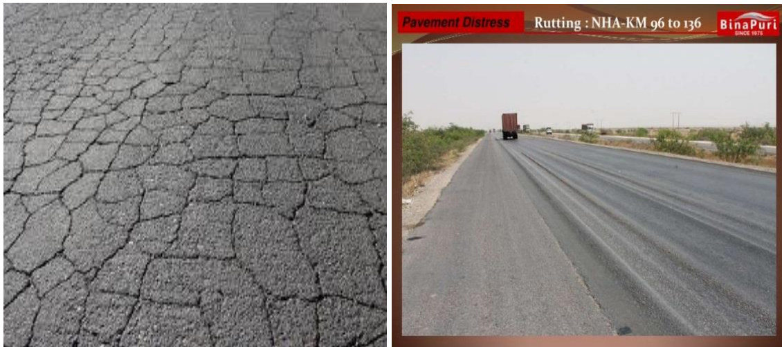
Figure 2.2 Fatigue and Rutting Pictures in Pakistan
