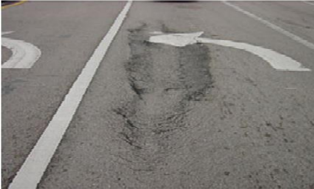
Figure 2: Slippage Crack in Turning Area
