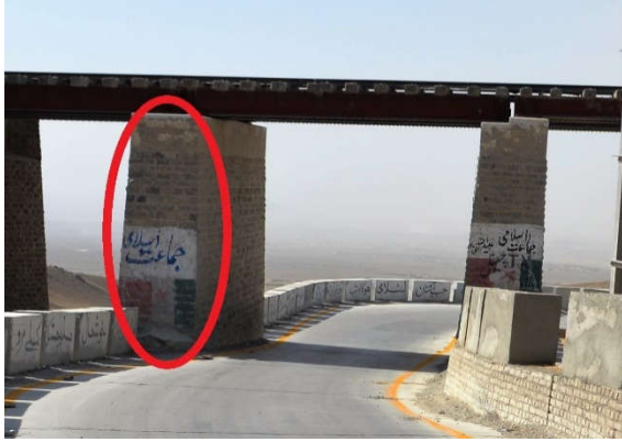
Figure 4.28-Illustrates fixed object at section (Non-project)
