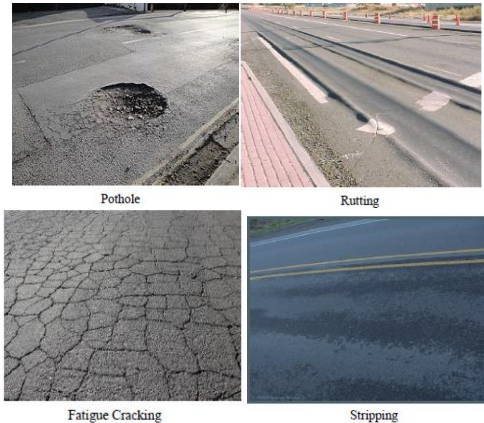
Figure 2. 7: Moisture-induced damage (online source)
