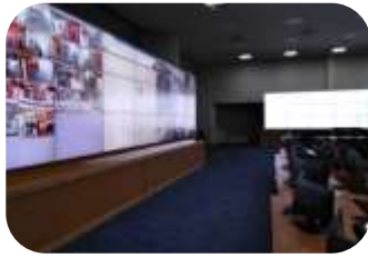
Video Surveillance Wall of C&CC
