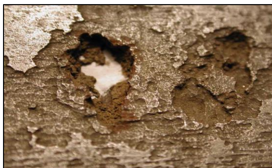
Figure 2-10; MIC corrosion on heating oil tank [44]
