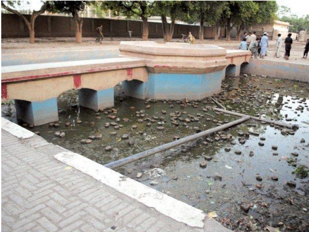
Figure 5 Condition of Fountain in Wazir Bagh
