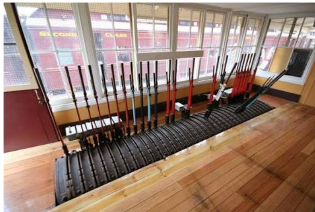
Figure 1.10: Mechanical Interlocking in Pakistan Railway [45]
