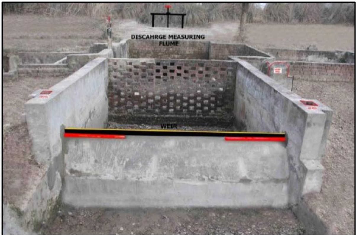
Figure 4.3: Discharge measuring flume
