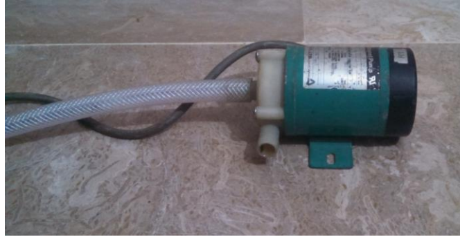
Fig 3.2: Chilled water circulating pump-2 with 960 L/Hr flow rate
