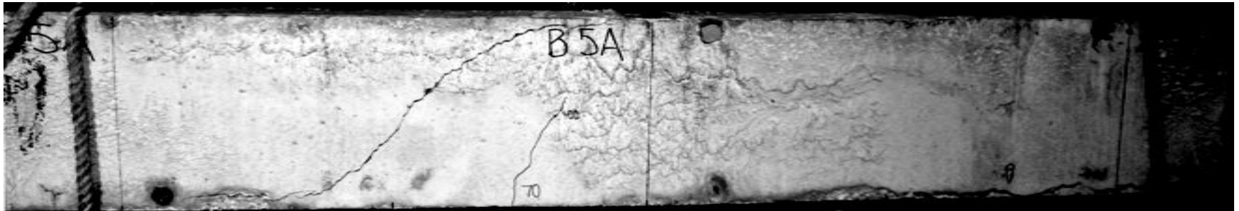
Fig 4.6 Crack Pattern of Beam B5A
