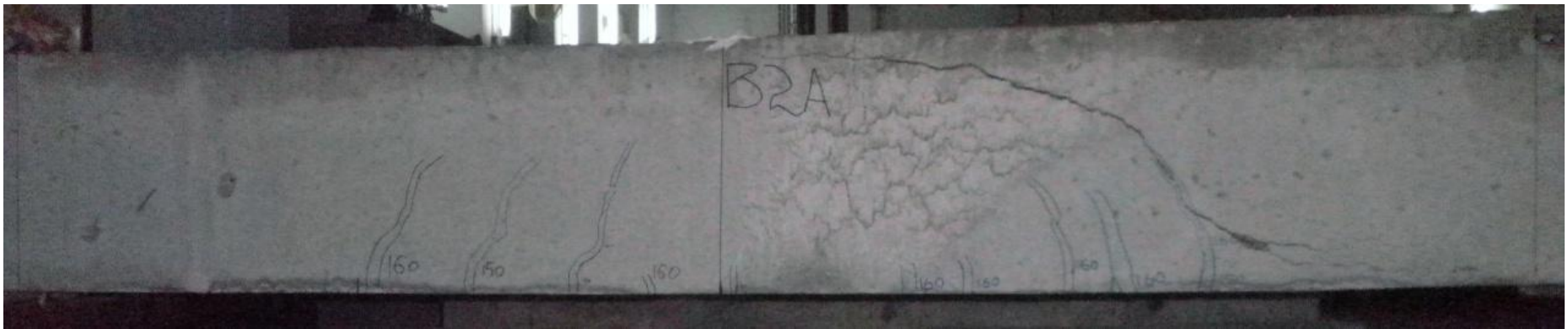
Fig 4.6 Crack Pattern of Beam B2A
