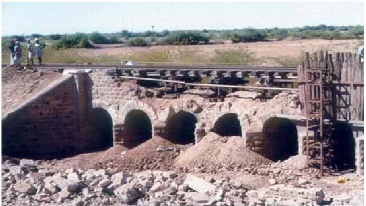
Figure 2.8: Overturning of the walls for a transport masonry bridge, after the Bhuj earthquake, 2001, India [Gisdevelopment, 2001]
