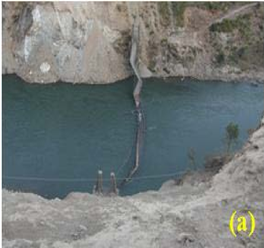
Figure 2.7: (a) Collapse of a suspension bridge over River Neelum due to landslides
