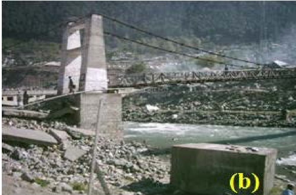
Figure 2.7: (b) Slippage of side-sway cable anchor block & failure of approach road to bridge.[S.M.Ali, 2009]
