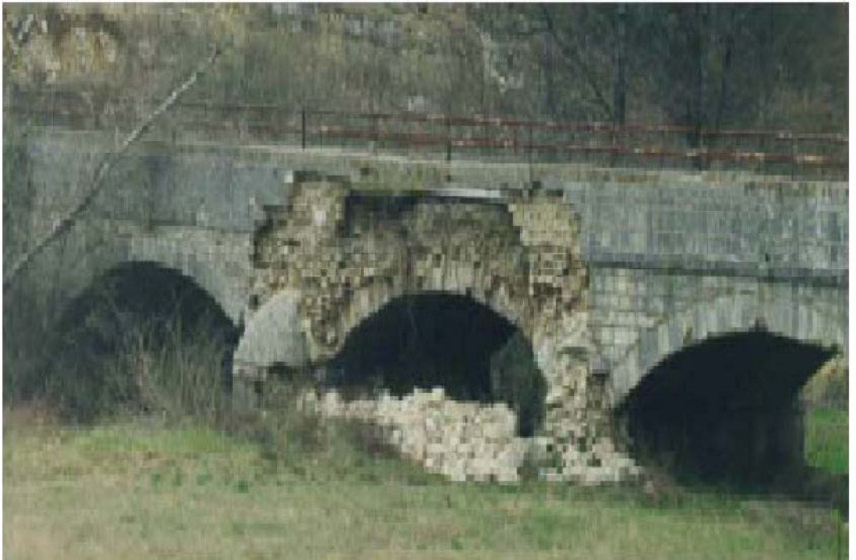
Figure 2.9: Damage of a masonry bridge, after the Umbria-Marche earthquake, 1997 [Resemini and Lagomarsino, 2004]
