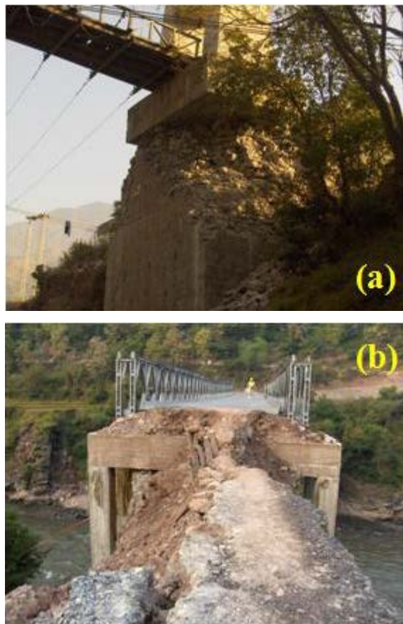
Figure 2.6: (a) Severe damage to the stone masonry base of tower in a suspension bridge (b) Collapse of stone masonry retaining wall that resulted in failure of approach road.
