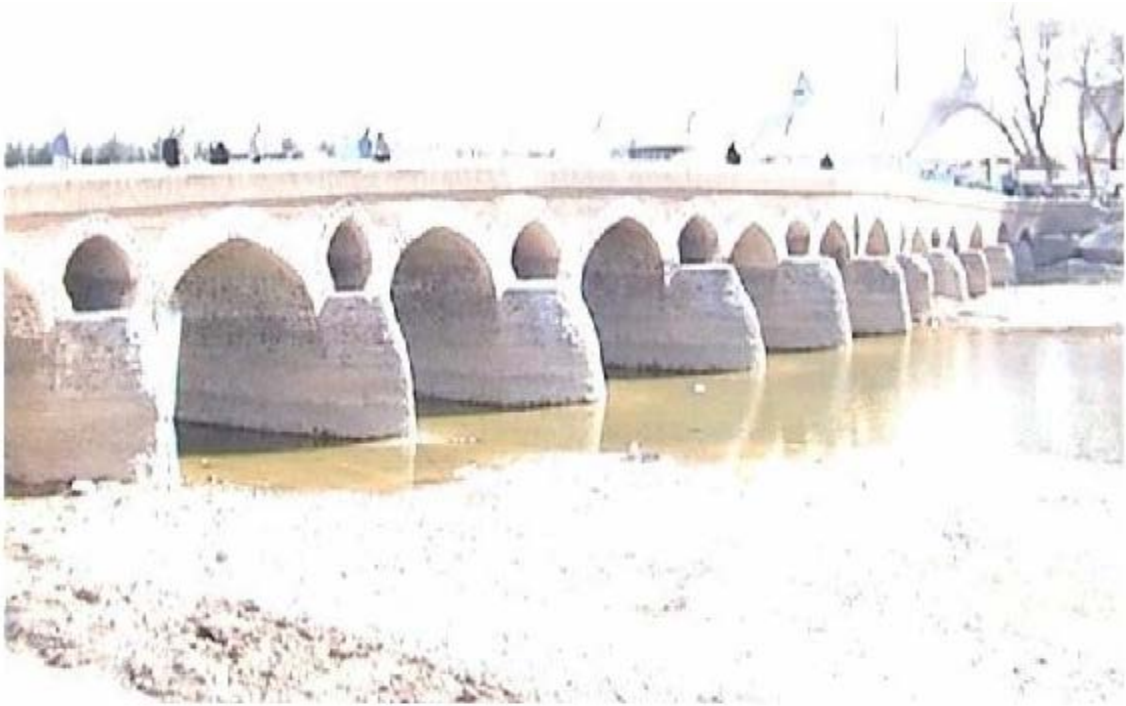
Figure 1.1: Shahrestan Bridge (twelfth century) on the Zayande River: Mixed masonry (stone blocks and bricks), 100m span and 11 arches
