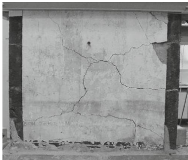
Figure 4.38 Cracking pattern under 2nd cycle of loading
