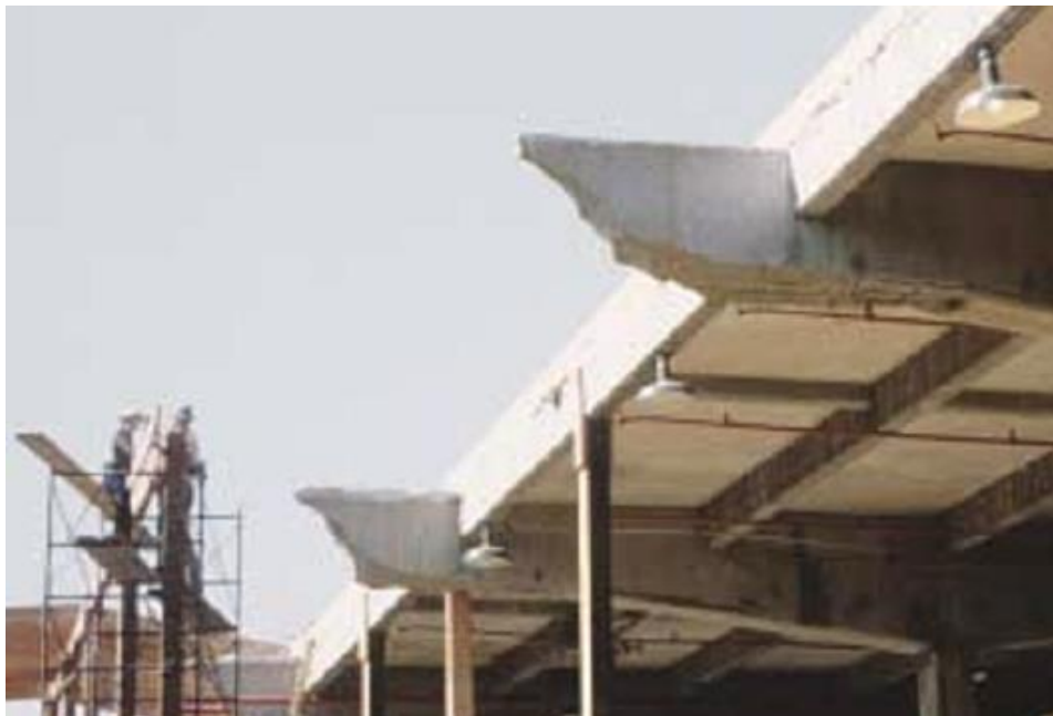
Figure 1.2: Shear failure of 36-in deep beams in air force warehouse, Shelby, Ohio USA (Lubell et al. 2004).
