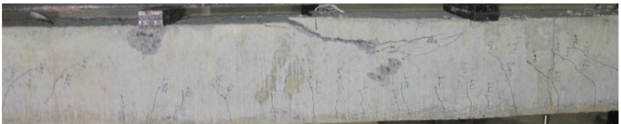
Figure B-31 : Typical failure of Confined Beam (Spalling of cover)
