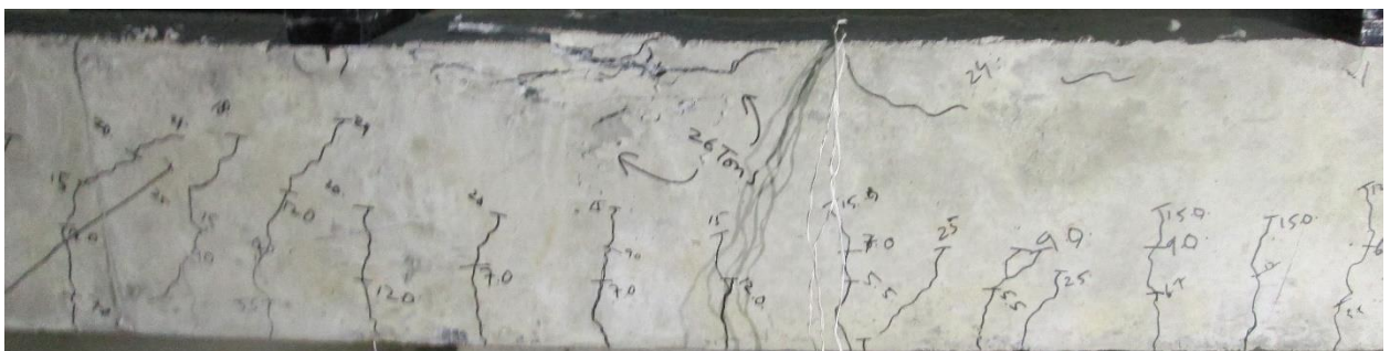
Figure B-28 : Cracking Pattern of R-OR-2
