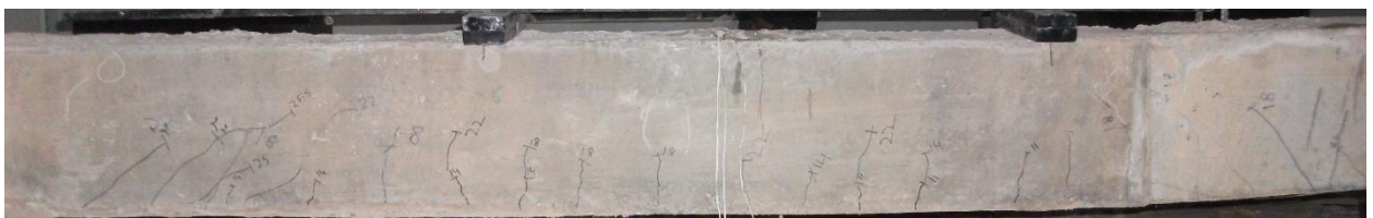
Figure B-21 : Cracking Pattern of R-OR-1
