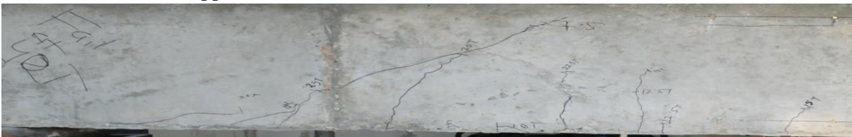
Figure 0 7: Cracking Pattern A-1
